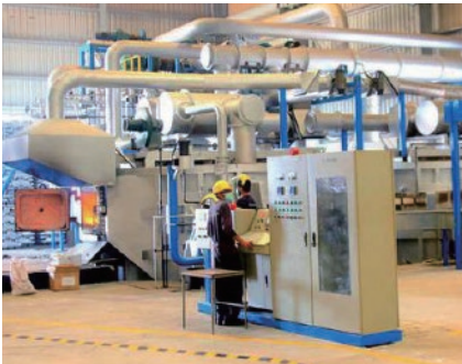
Pakistan Cables Nooriabad Factory (Pakistan)
